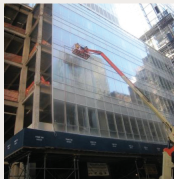
Figure 30: Calibrated sprinkler rack hung from a motorized man lift
