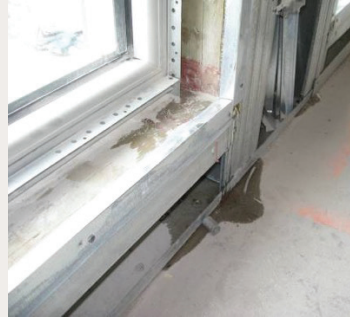
Figure 6: Example of water infiltration at a punch window assembly
