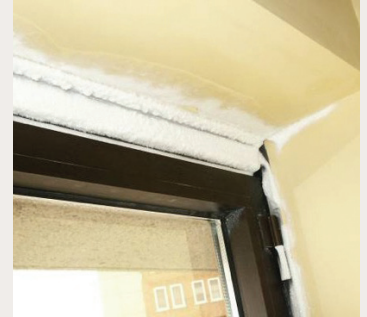
Figure 8: Example of excessive interior frost formation due to excessive air infiltration at a window/wall interface
