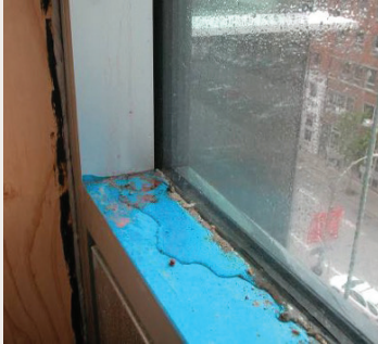
Figure 5: Example of water infiltration within a curtain wall assembly
