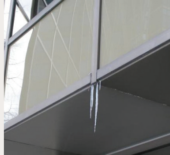
Figure 7: Example of exterior icicle formation due to excessive air exfiltration within a curtain wall assembly
