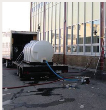
Figure 31: Portable water reservoir and pump system
